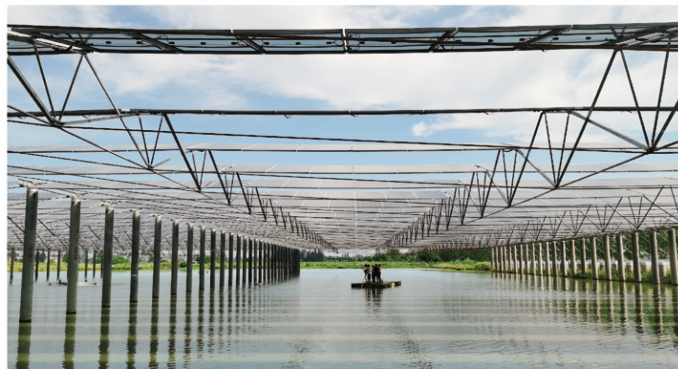
湖北洪湖200MW柔性支架渔光互补电站 Hubei Honghu 200MW Fishery-Photovoltaic Complementary PV Power Plant
