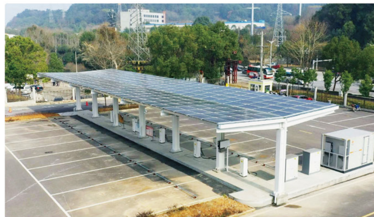
湖北黄石客运枢纽站光储充电站 Hubei Huangshi Passenger Transport Hub PV-Storage-Charging Station
