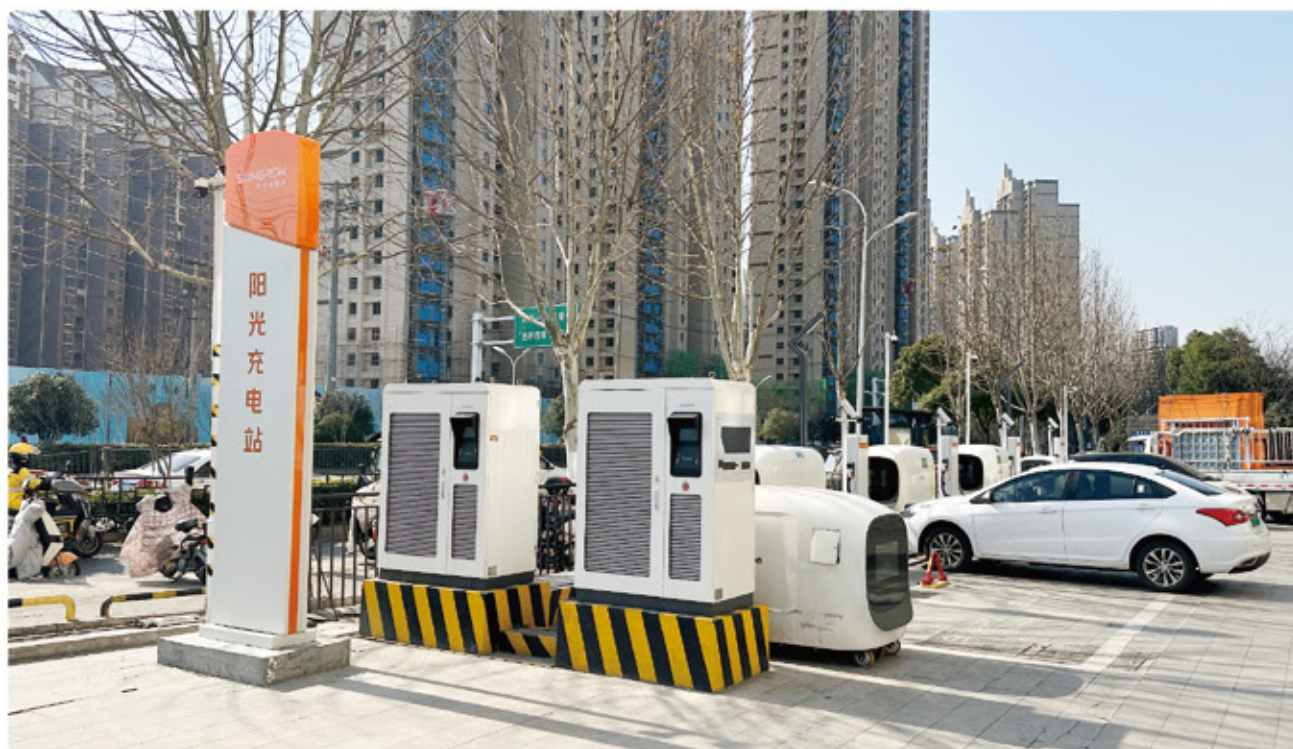
安徽合肥神力商业中心充电站 Anhui Hefei Shenli Commercial Center Charging Station
