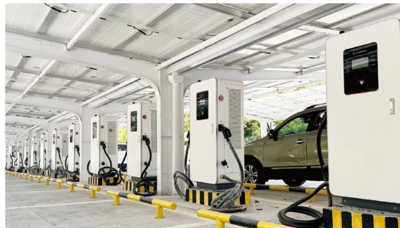
重庆首座零碳服务舱光储充电站 Chongqing's First Zero-Carbon Service Pod PV-Storage-Charging Station
