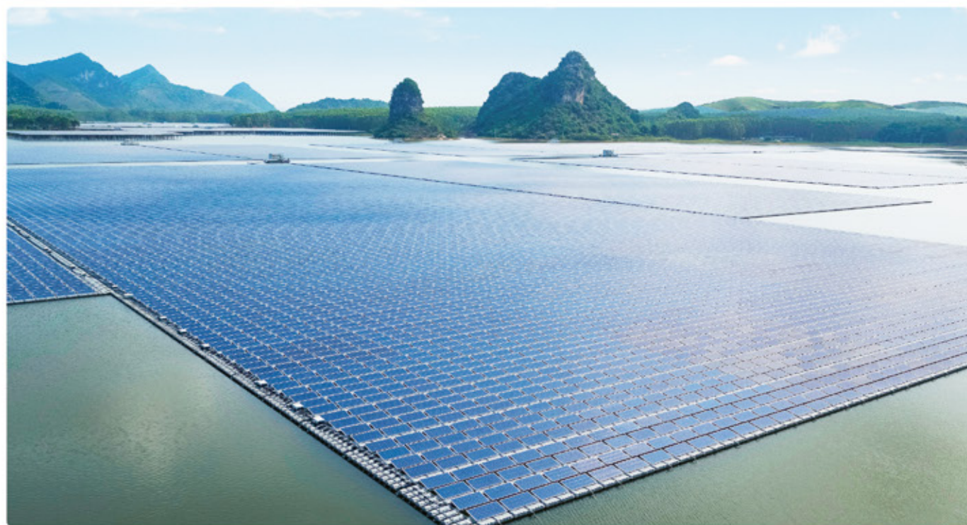
广西覃塘古平水库40MW漂浮电站 Guangxi Qintang Guping Reservoir 40MW Floating PV Power Plant
