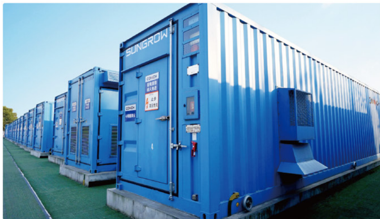
首批科技创新（储能）试点示范项目——张家港海螺水泥厂8MW/32MWh工商业储能电站 First Batch of Technology Innovation (Energy Storage) Pilot Project - Zhangjiagang Conch Cement Plant 8MW/32MWh Commercial Energy Storage Power Plant
