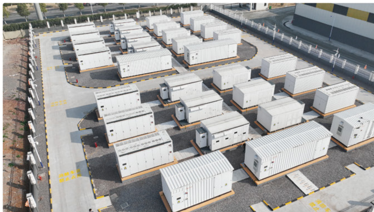
安徽友进冠华35MW/70MWh工商业储能电站 Anhui Youjin Guanhua 35MW/70MWh Commercial Energy Storage Power Plant
