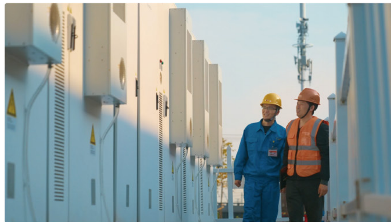
浙江温州人本轴承1MW/2.15MWh工商业储能电站 Zhejiang Wenzhou Renben Bearing 1MW/2.15MWh Commercial Energy Storage Power Plant
