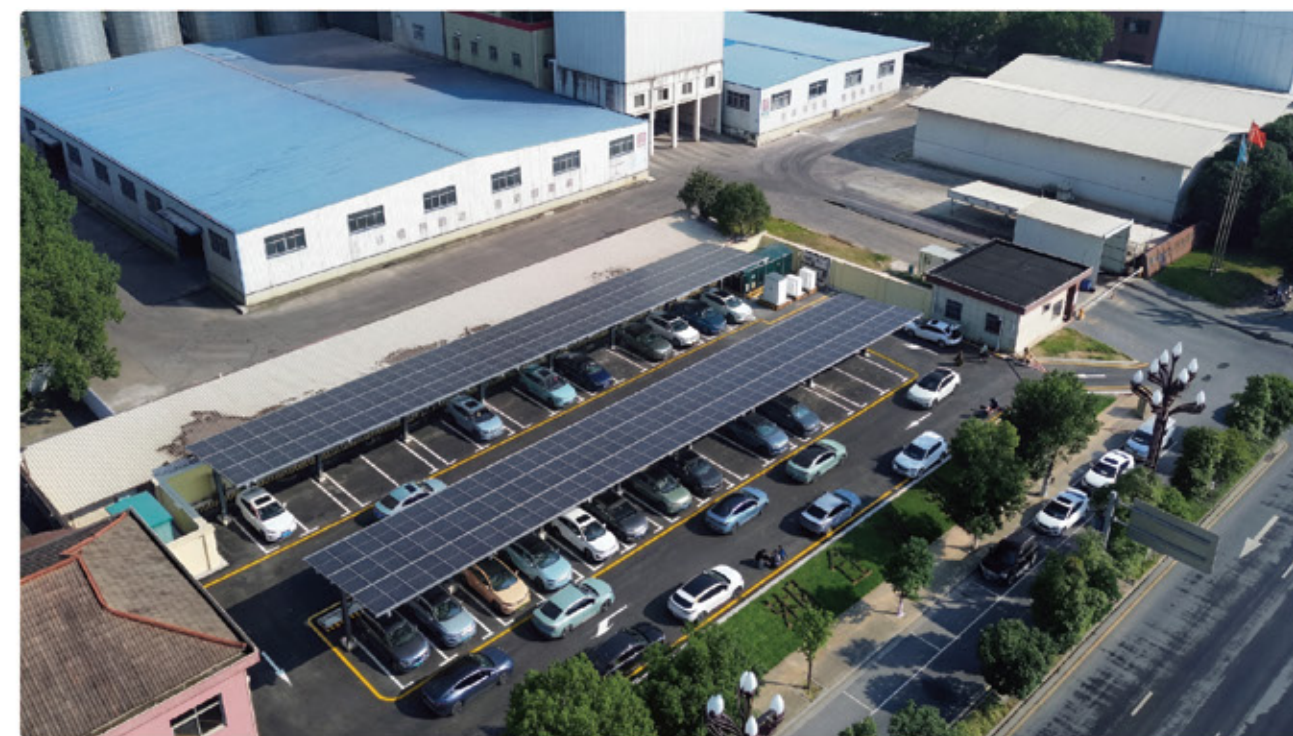
湖南常德光储充电站 Hunan Changde PV-Storage-Charging Station
