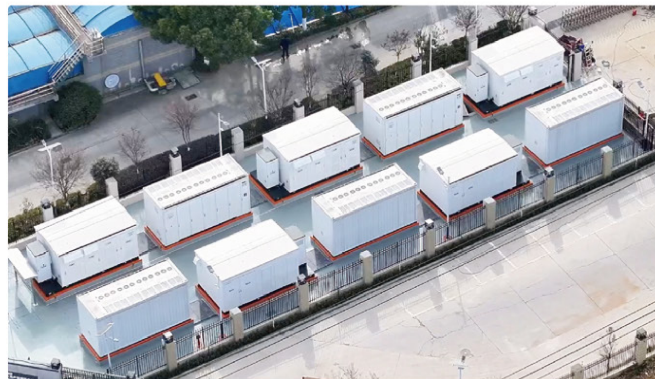
安利股份12.5MW/25MWh工商业储能电站 Anli Group 12.5MW/25MWh Commercial Energy Storage Power Plant
